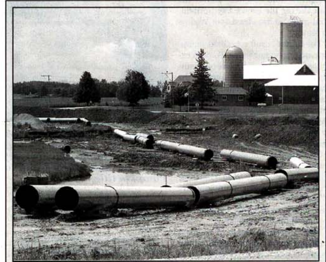
PIPELINE PROCEEDS – Although not all of the legal issues raised by affected landowners have been resolved, construction goes on in east central Wisconsin for the 120-mile natural gas pipeline being installed for Guardian Pipeline. This scene is at U.S. Highway 151 and Town Hall Road, west of Chilton in Calumet County. (Photo by Ray Mueller)
